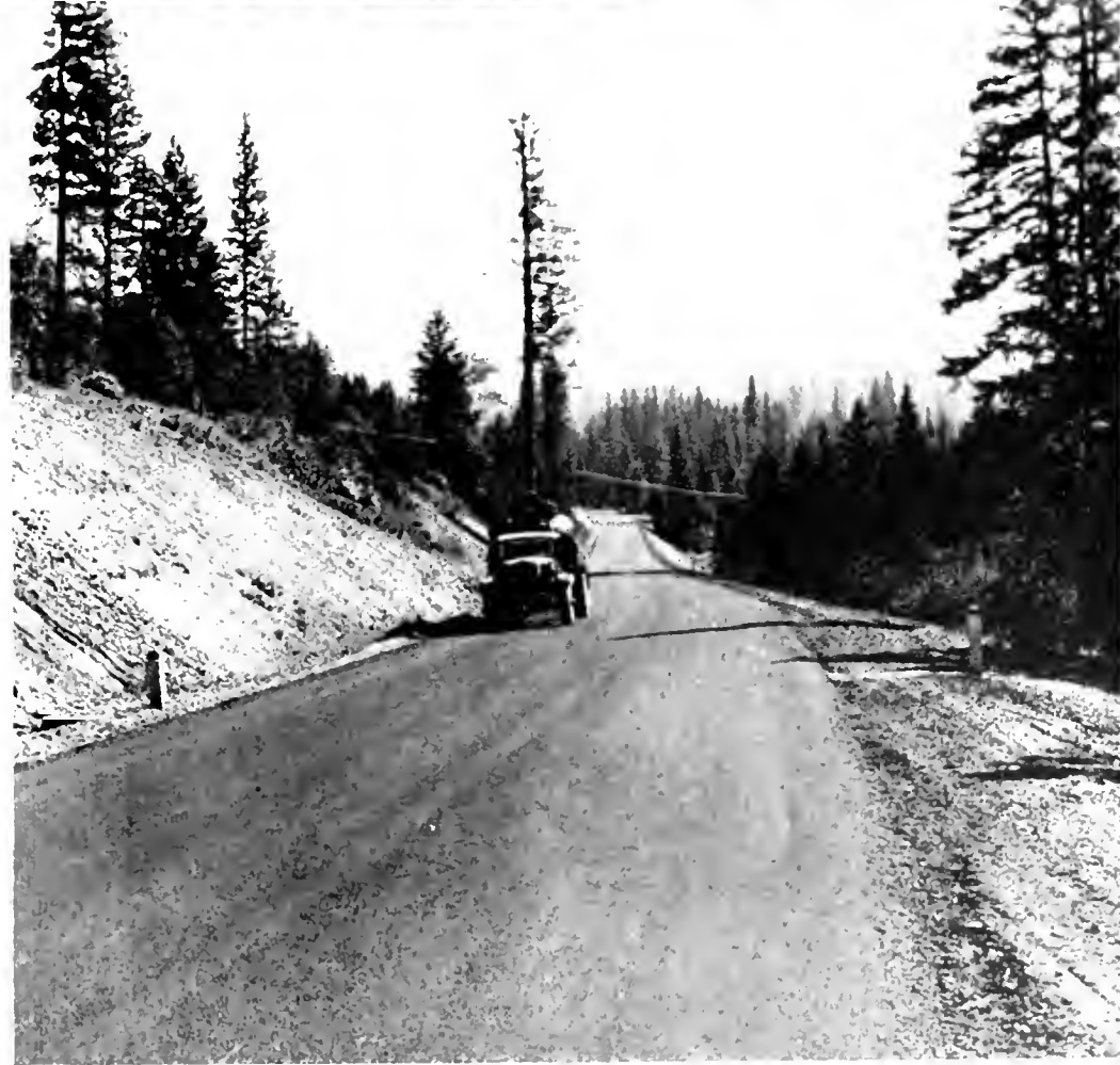
Above—Completed highway near Keddie. Below—load of logs being hauled from mill on another section of new highway
